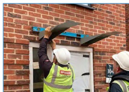
5. Level bracket with spirit level and if require pack to required position.
